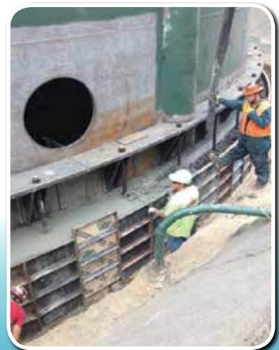
Pouring concrete in the support foundation at the View Acres water reservoirs seismic upgrade.
