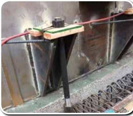
2013/14 seismic upgrade to the Oak Lodge Water District View Acres water reservoirs.
